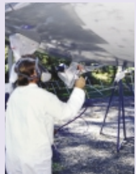
An epoxy barrier coat sprayed on a newly relaminated surface can stop further water permeation.
